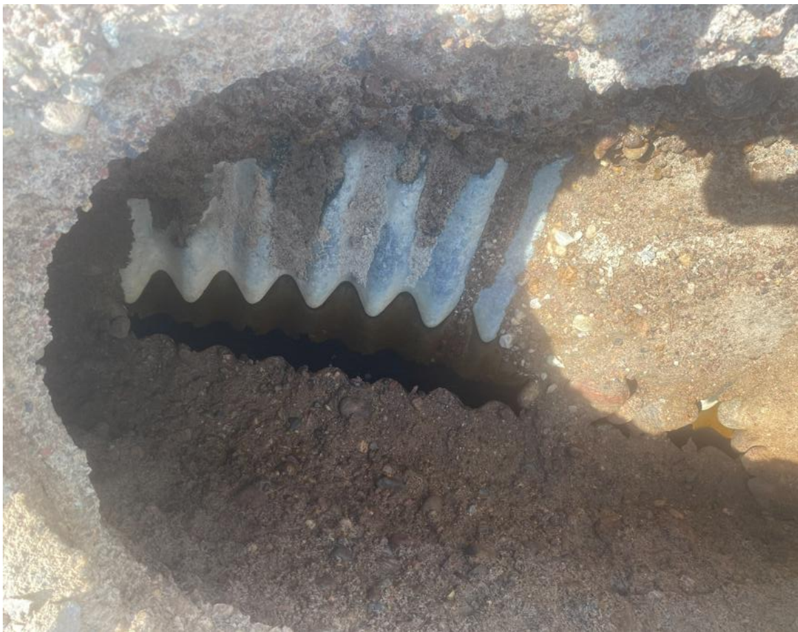
Open hole of failed multiplate (current picture)
