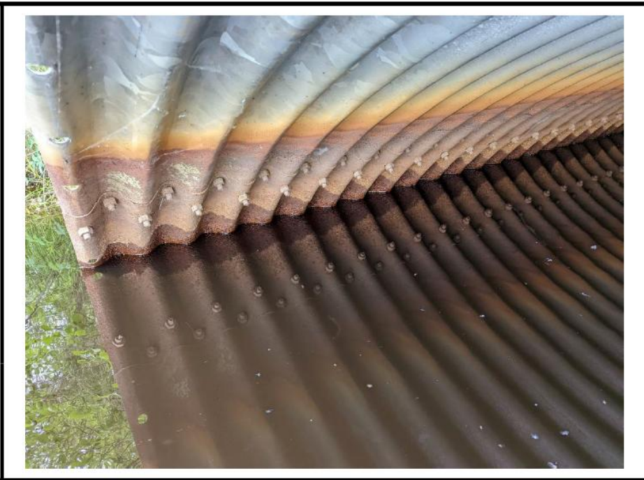
Photo 8 Light to moderate corrosion noted at and above waterline
